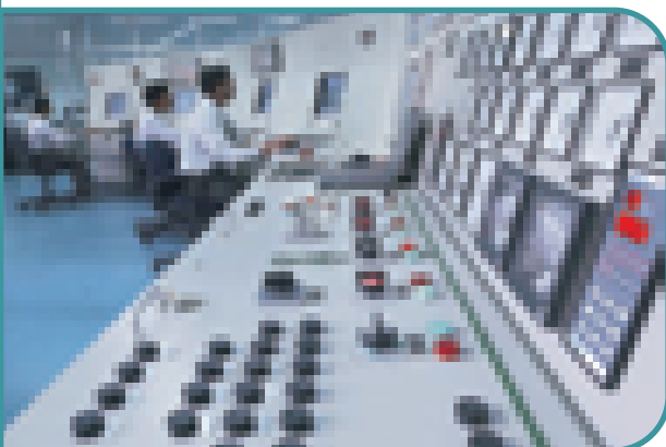
Cutting-edge technology provides a good platform for our employees to excel. Shown here, the Control Room.
